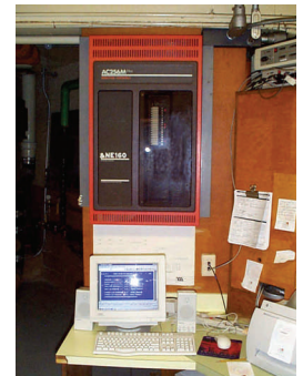
The Energy Management Computer watches for heat and cold around the clock
