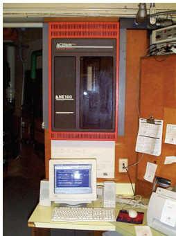
The Energy Management Computer watches for heat and cold around the clock
