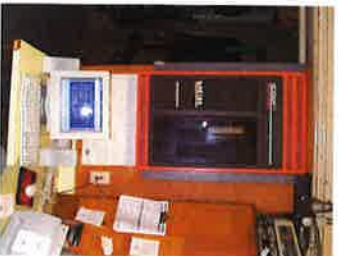
The Energy Management Computer watches for heat and cold around the clock
